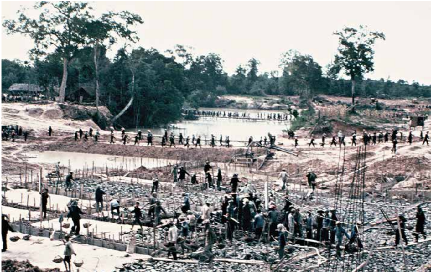
Irrigation dam construction on the road north in 1978. Photo by Gunnar Bergstrom. For fourteen days in 1978, Bergstrom and other members of the Swedish Cambodian Friendship Association undertook a “public relations” tour choreographed by the Khmer Rouge, whose intention was to use the Swedes to rally support for the Khmer Rouge from abroad—particularly from other communist countries. A collection of Mr. Bergstrom’s photos during the trip was published in a book titled, “Living Hell.” (Gunnar Bergstrom/ Documentation Center of Cambodia Archives)
